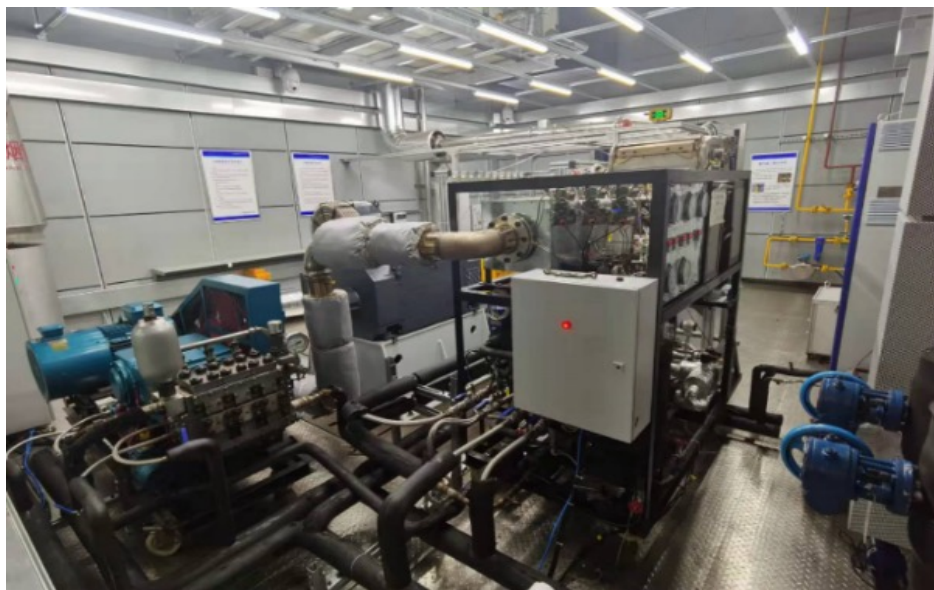
sCO 2 跨临界动力循环样机 The sCO 2 power cycle test bench
