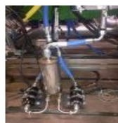
储液罐及工质泵 tank and pump
