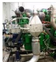
烟气换热器 Flue gas heat exchanger
